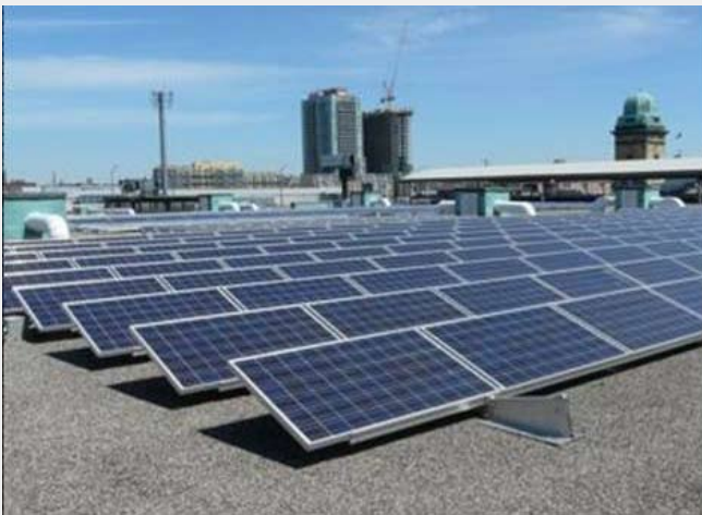
Figure 81.3 Renewable energy solar PV panels
